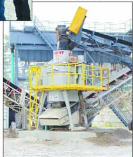
The REMco SandMax 250 VSI crusher was purchased in January, installed by Hylka personnel and put into service in mid-June.
